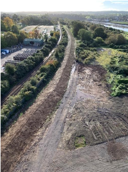
Photo 1 – Lamplighter’s Marsh. New earth embankment in front of railway as part of ASEA Project.
